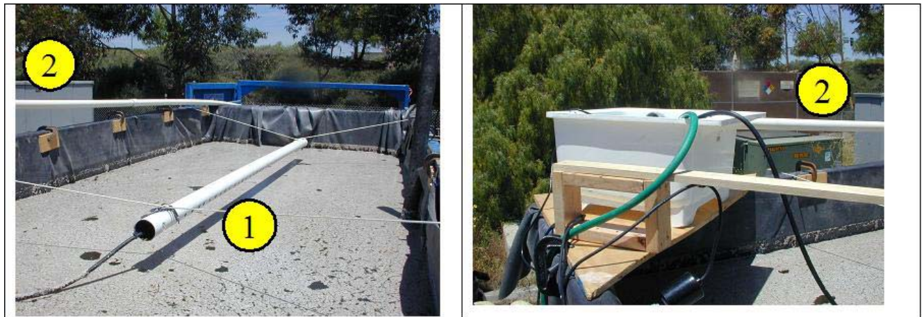
Figure 11: The metering tank had a submersible pump connected to a float valve.
